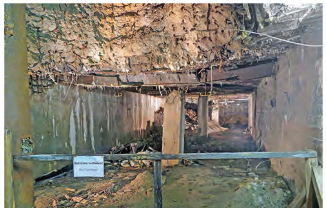
The damage resulting from the partial demolition of Zeppelin. The loss of useable space made little difference to the reusability of this massive bunker. Photo Clive Penfold
